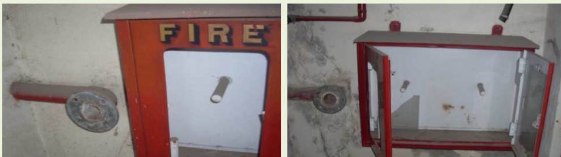
Defunct Hydrant system in Gagan Vihar (12 July 2012)
